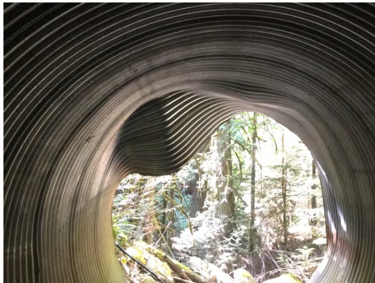
Damage to outlet
